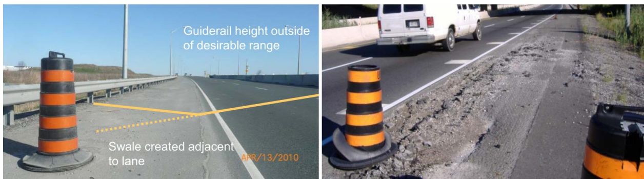
Figure 37. Highway 427 – Guiderail Height Outside of Desirable Range and Swale Created Adjacent to Lane (2010)
