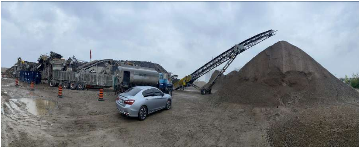
Photo (17): Crupi Crusher at 176 Bethridge Rd, Etobicoke, ON – Producing RCA
