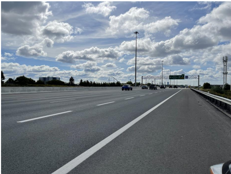
Figure 21. Highway 400- Southbound Direction Before Exit to Major Mackenzie Drive - No Distresses (September 2022)
