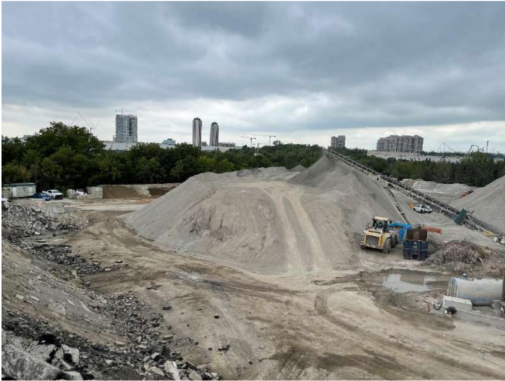
Photo (9): Strada Crusher at 1667 Creditstone Rd, Concord, ON – Stockpile of RCA (Gran A RAP)
