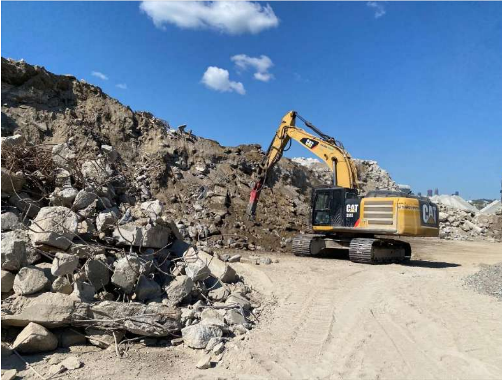
Photo (31): Strada Aggregate Crusher: 10 Leslie St, Toronto, ON Breaking Big Pieces of Concrete Prior Crushing
