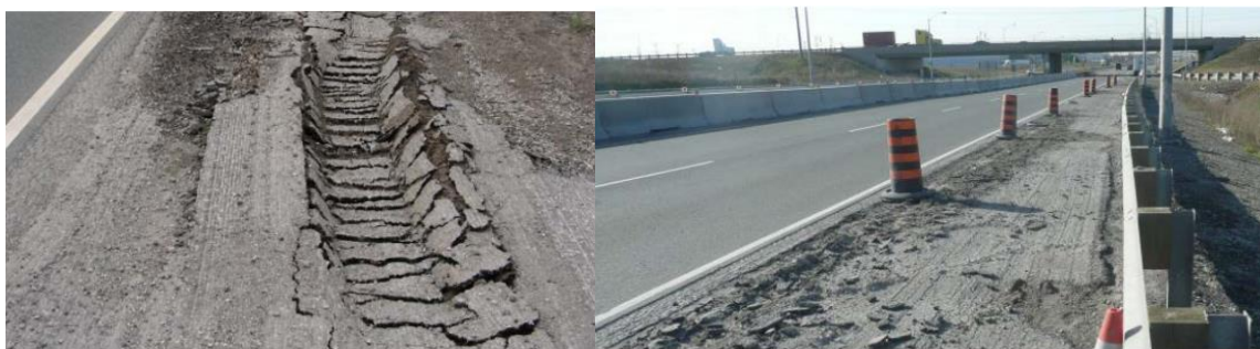
Figure 38. Highway 427 – Different Pavement Distresses (2010 -2011)
