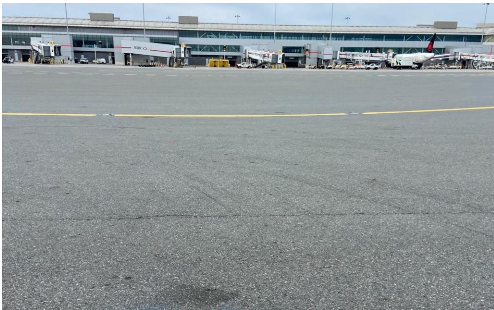
Figure 16. Pearson International Airport – T1 Apron Asphalt, Occasional Construction Joint Cracking in Slight to Moderate Severity. Occasional Asphalt Raveling in Slight Severity (EXP - November 2021)
