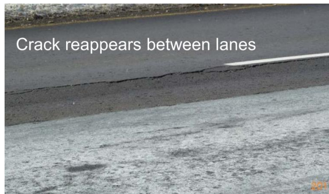
Figure 35. Highway 427 – Reappearance of Cracks Between Lanes in 2011
