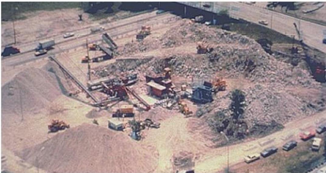
Figure 22. Concrete Recycling Operation Set up Inside of Edens Expressway Cloverleaf Interchange (Photo from NHI 1998) [13]
