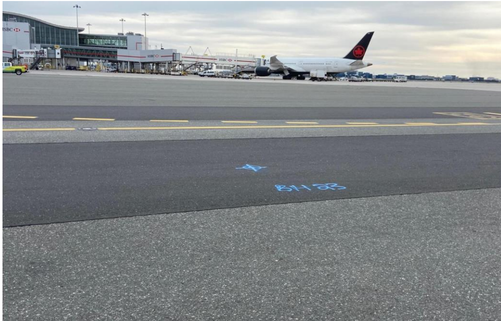
Figure 15. Pearson International Airport – T1 Apron Asphalt Observed Patches in Fair Condition (EXP - November 2021)
