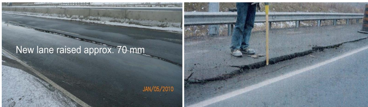
Figure 34. Highway 427 – Pavement Heaving in 2010
