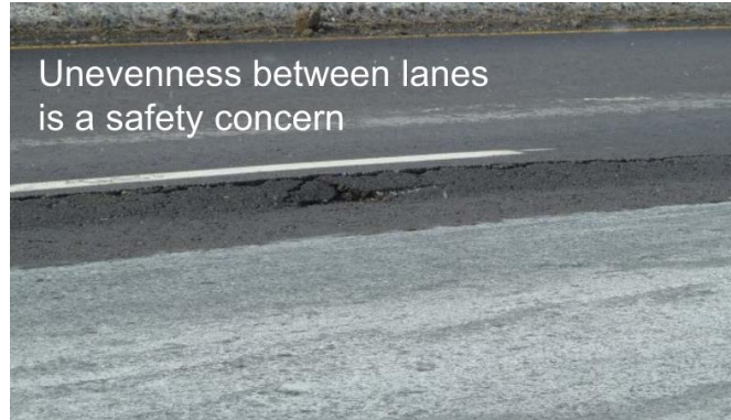
Figure 36. Highway 427 – Pavement Distresses Between Lanes in 2010 - 2011
